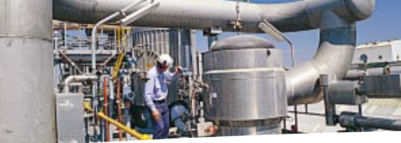
Reading the vacuum system pressure transmitter on Incitec's new urea granulator plant at Gibson Island (Queensland, Australia)
