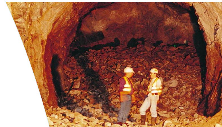
Orica's technical expertise is the key in the successful tunnelling project in Hong Kong.
