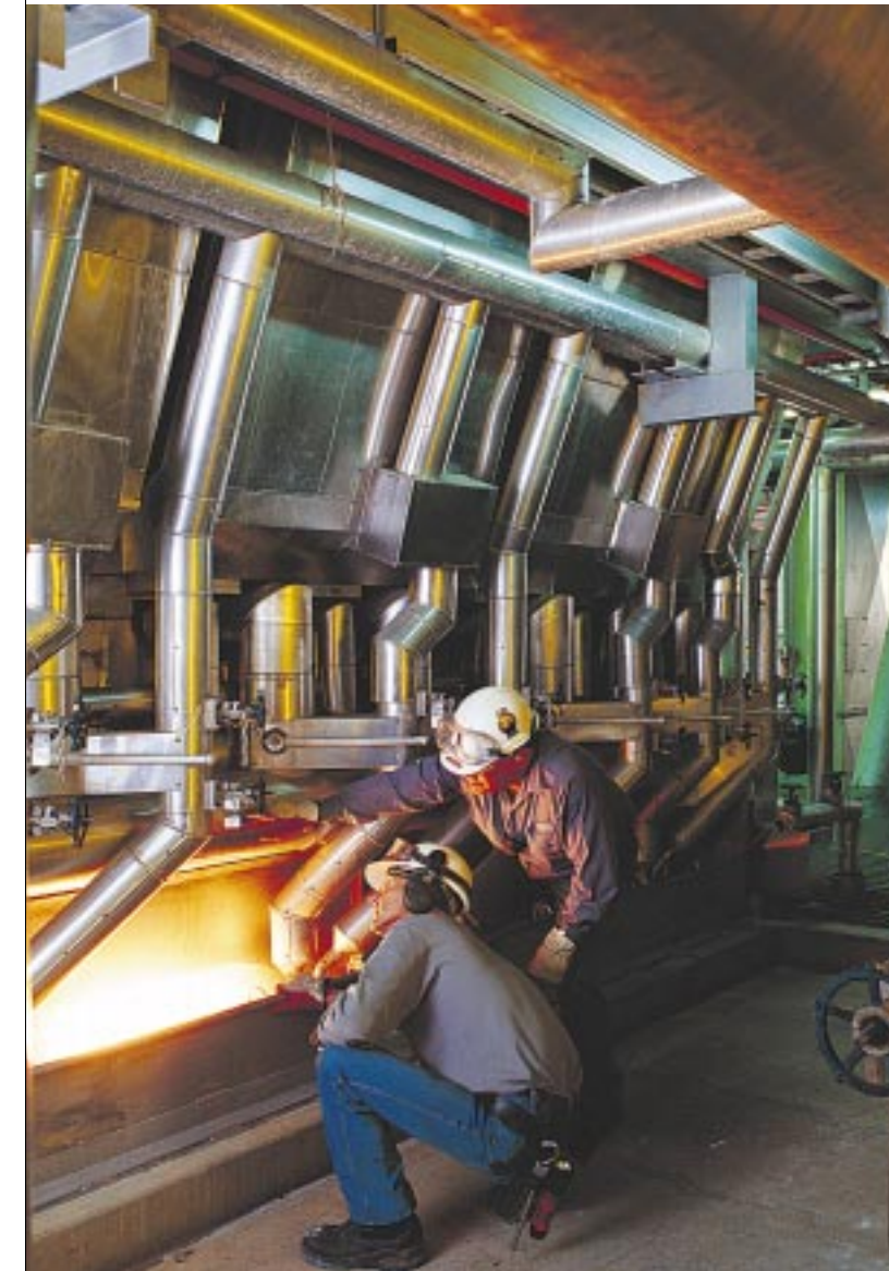
Plant Technicians Steve Humalisto (left) and Allister Powell at the granulator melt headers in the new urea granulation plant at Gibson Island (Queensland, Australia)
